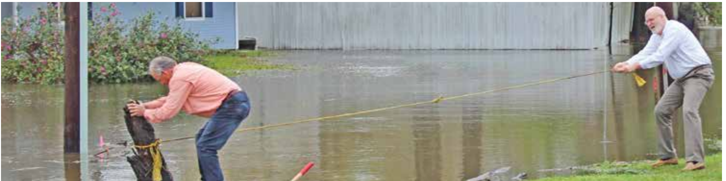
Before the flood: city staff and residents have ample experience with typical flood conditions. In this March 2016 photo, IBTS Program Director David Ratcliff (l) and Mayor Jr Shelton (r) help clear debris from a culvert. Photo credit: Jolice Provost, Central City News.
